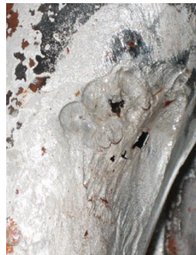
Fig. 3 Corrosion of bent tube near burner
