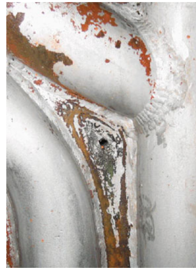
Fig. 2 Corrosion of irregular fin near burner
